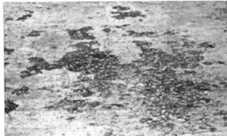
Scaling concrete surface
